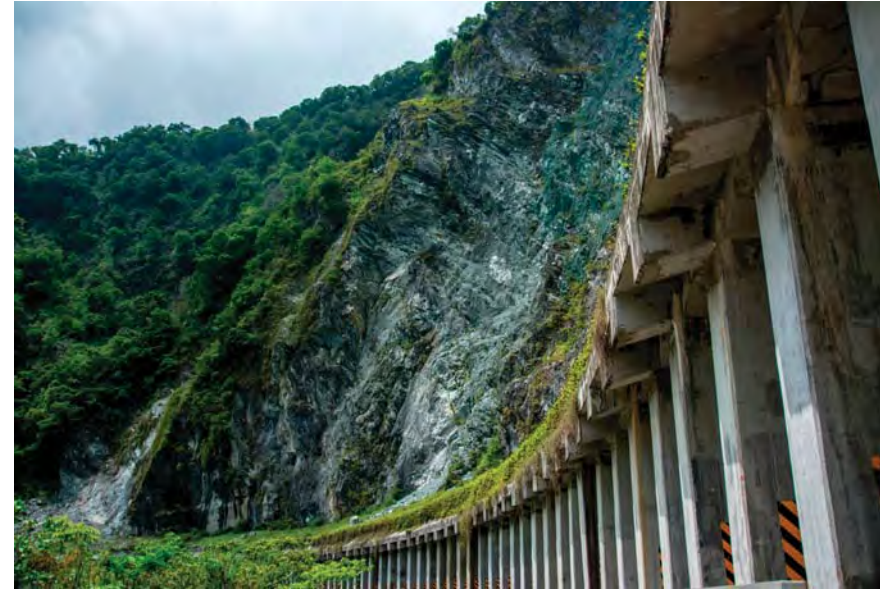
Landslide to the east of Tai Shan Tunnel.
